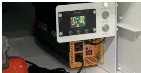
Onboard power systems
